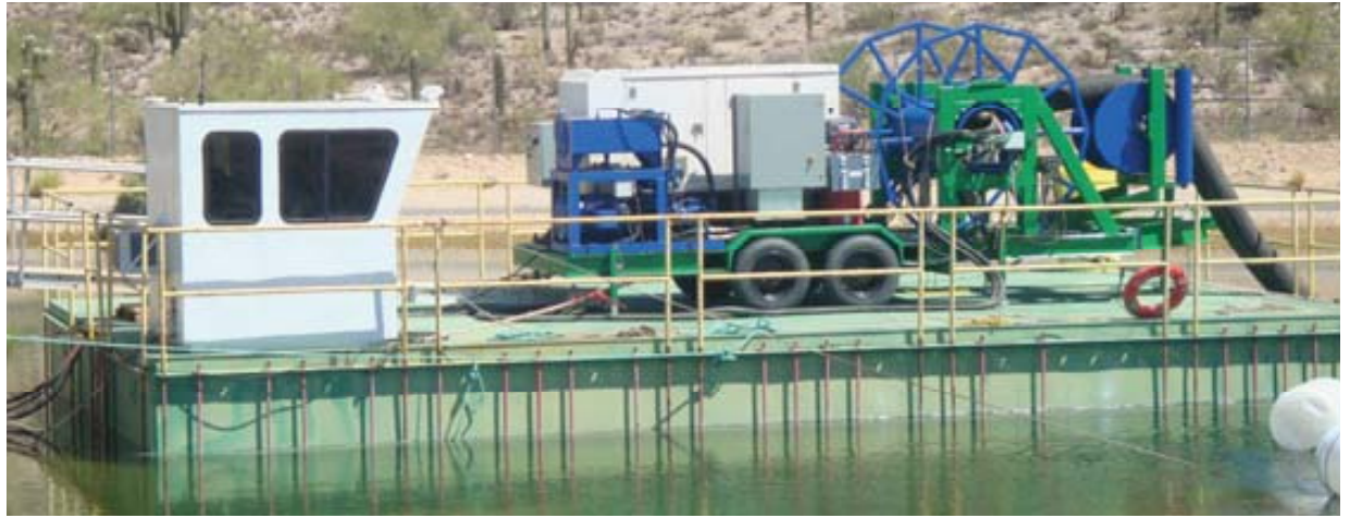
Expected to start in February, a special pump will be mounted on a barge to carefully remove sediment from the bottom of the Singh reservoir.
